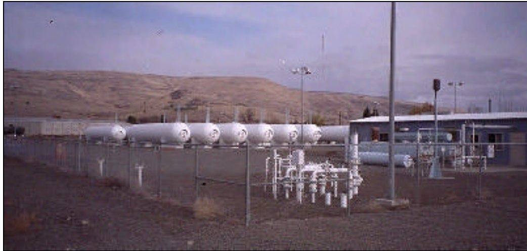
Large Propane-Air Peakshaving Facility
