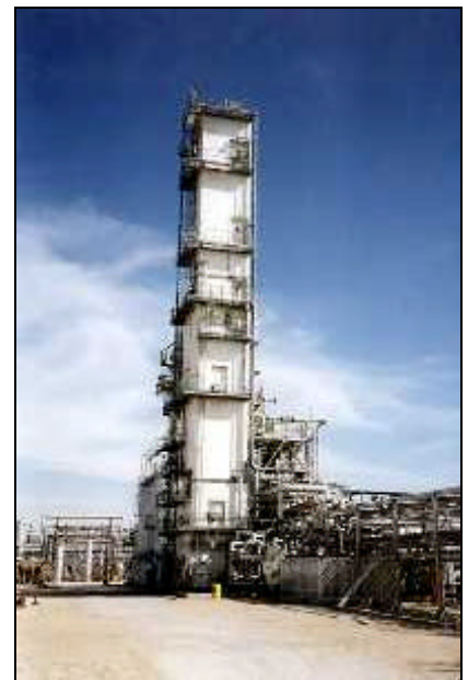
Nitrogen Rejection Unit
